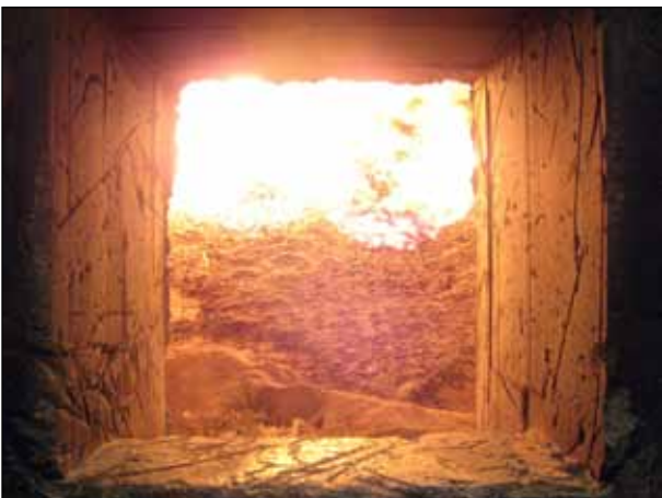
The boiler in action! Photos: DOF
