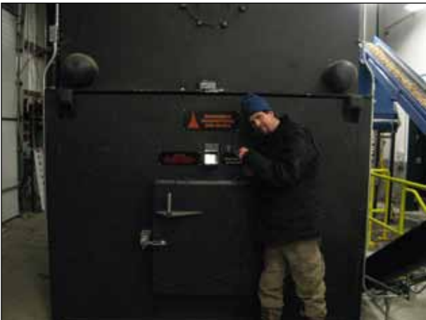
Hermanns and the boiler. Photos: DOF
